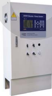
General Inverter within the panel
